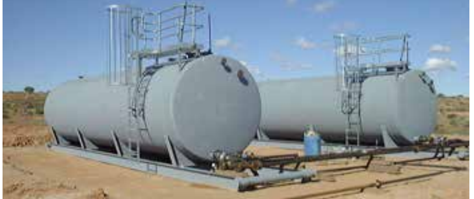
Storage tanks can develop moisture over time.
